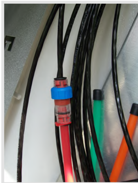
An example of placing a microduct system with the use of micro couplers
